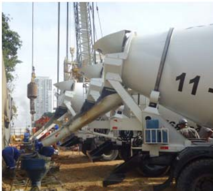
Figure 8. Concreting an initial panel with a length of 6.50m using multiple tremie pipes
